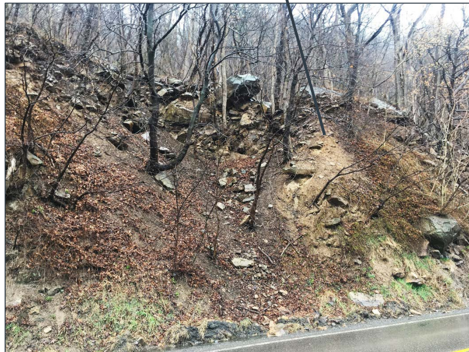
Rockfall Hazards Due To Erosion of Fines Allowing Boulders to Roll Out of Slope
