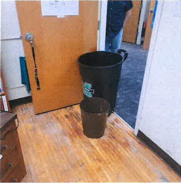
203D Office damage, caused by roof leak
