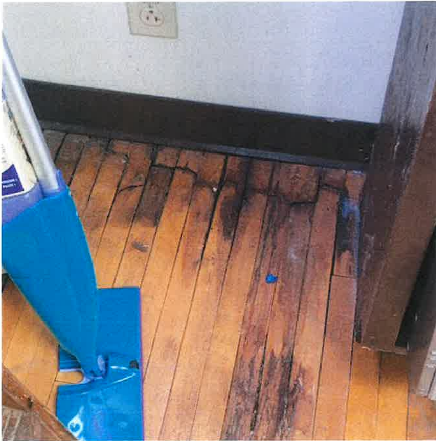
GH 203 – Classroom floor damage due to leaks
