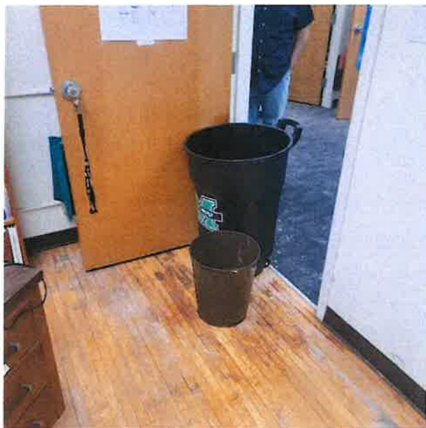
203D Office damage, caused by roof leak
