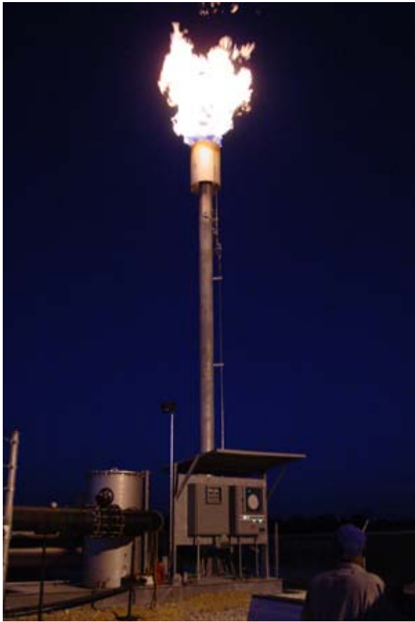
Landfill Flare in TX
