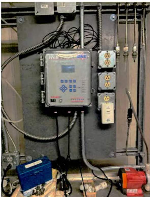
Engineering chemicals cooling tower
