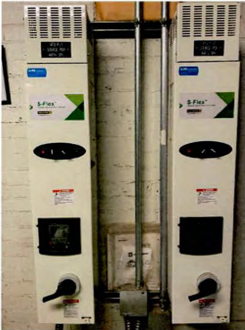
Education Building (Jenkins) 1 VFDs
