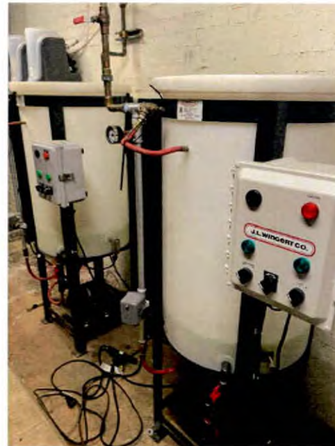
Education Building (Jenkins) 2 chemical tanks
