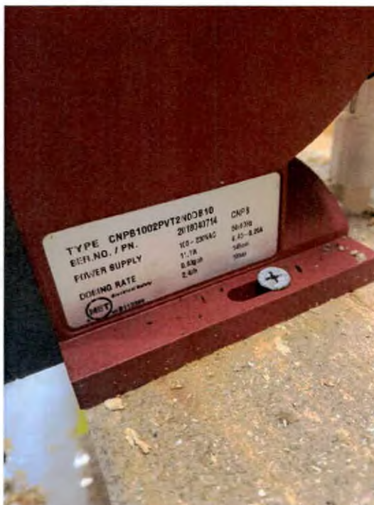
Old Main 4 chemical pumps close up
