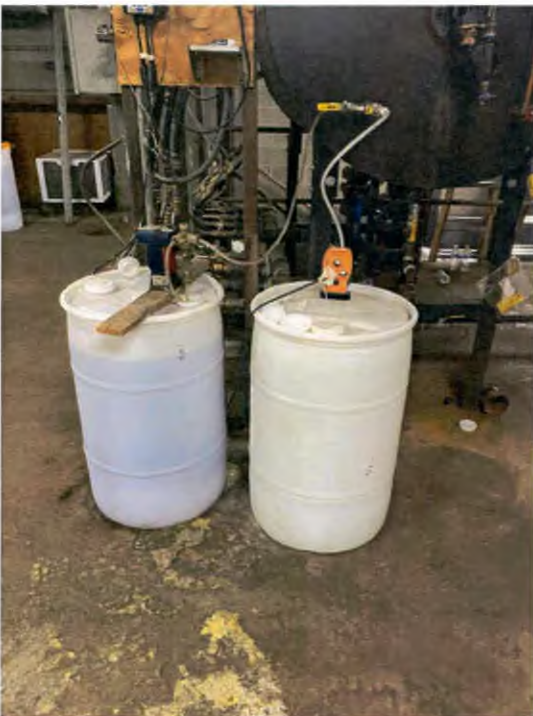
Henderson 1 chem pumps
