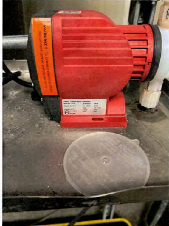
Biotech 2 chemical steam pump
