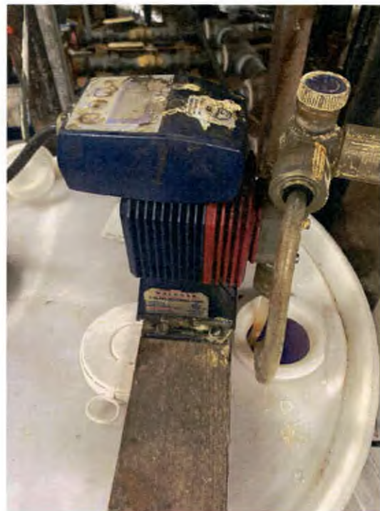
Henderson 2 chem pumps 2
