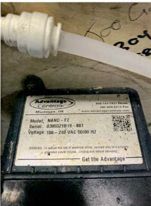
Old Main 3 chemical controller close up
