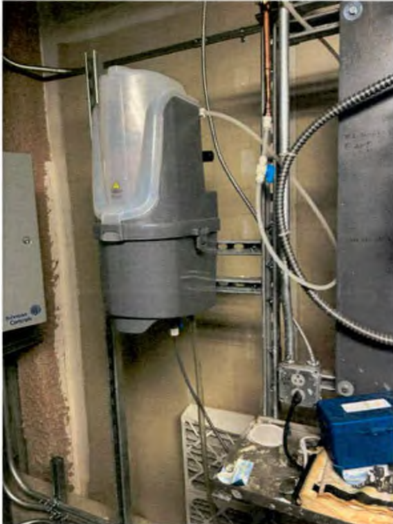
Biotech 1 chemicals steam dispenser
