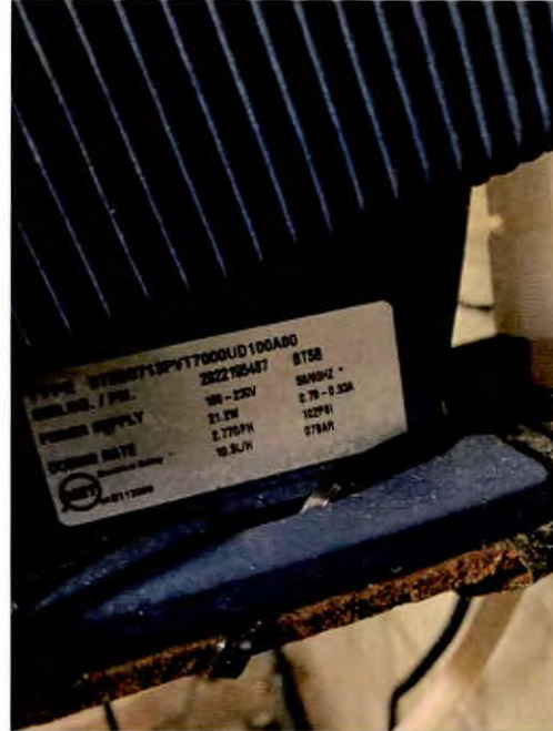
Drinko 6 chemical pump 2 close up
