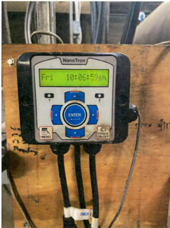
Henderson 3 chem pump controller
