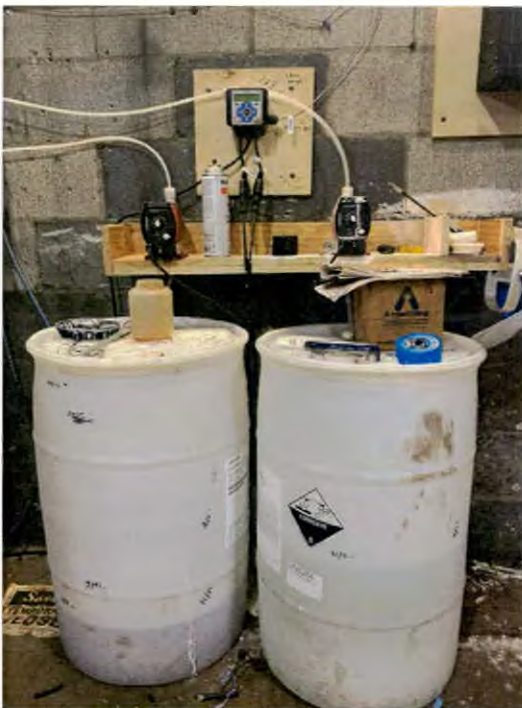
Old Main 1 chemical tanks
