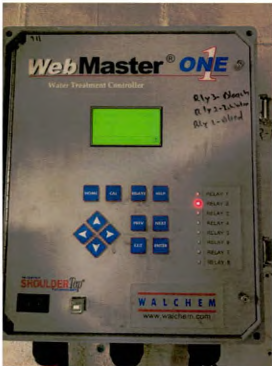
Science 1 chemicals controller
