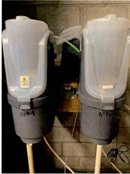
Drinko 2 chemical dispensers close up
