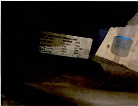
Science 5 chemicals pump 1 close up
