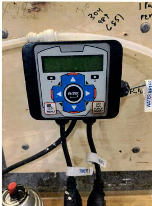
Old Main 2 chemical controller
