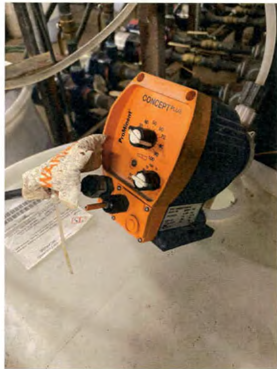
Henderson 4 chem pumps 1
