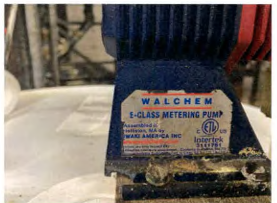
Henderson 6 chem pumps 2 close up
