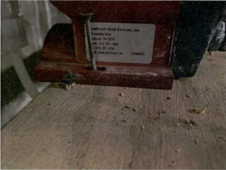
Fine Arts 8 chemical pump 2 close up
