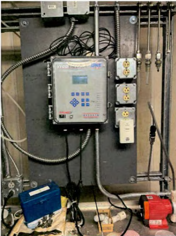
Biotech 3 chemicals cooling tower
