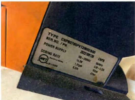
Henderson 5 chem pumps 1 close up
